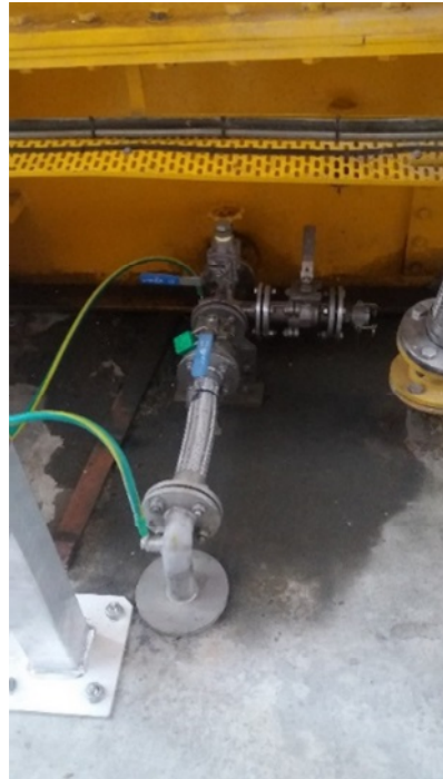
Figure 13: Drain valve transformer connection
