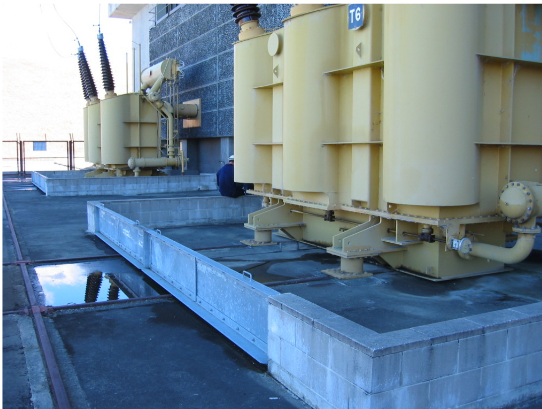
Figure 4: Old transformer bunds with steel gates
