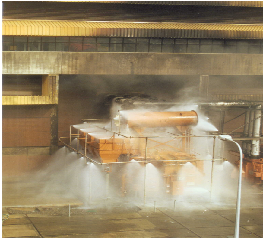
Figure 3: Huntly transformer fire with deluge system operating (O'Sullivan, 1999)
