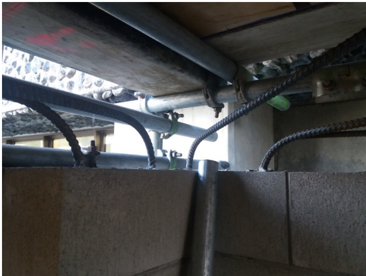
Figure 9: Bent reinforcing steel
