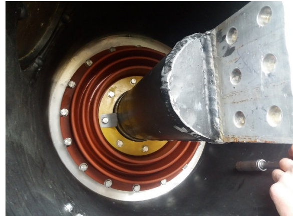
Figure 15: Fully installed oil barrier
