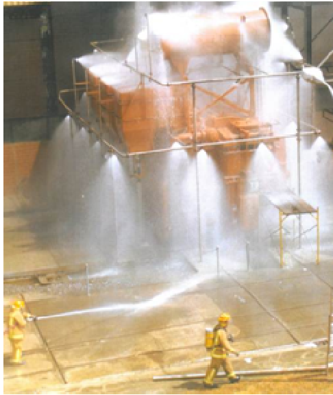
Figure 2 HVWS Sprinkler system in operation on a transformer
