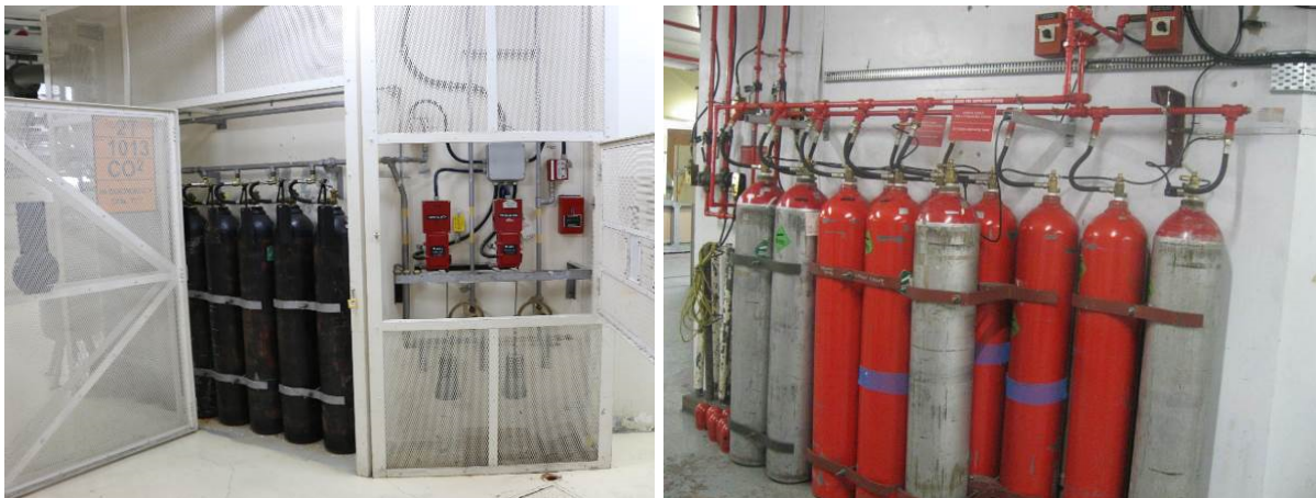
Figure 1: Typical existing CO 2 generator gaseous fire extinguishing systems.
