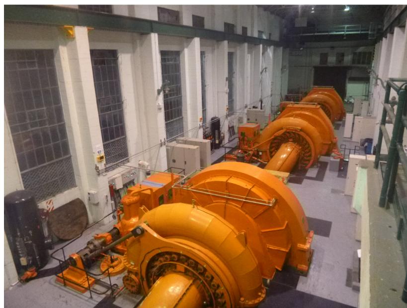
Figure 2: Tuai generators with hybrid system installed.
