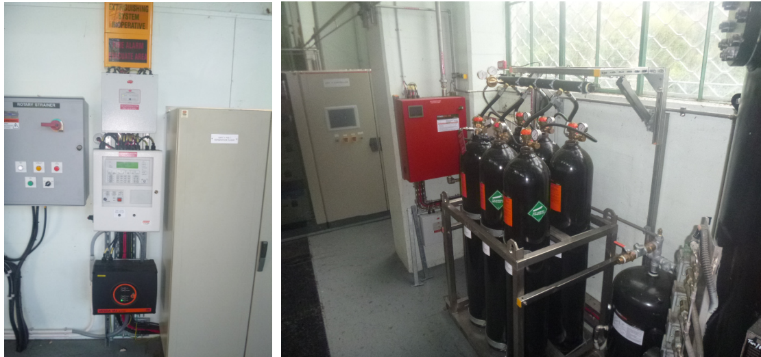
Figure 5: Controls and signage, discharge panel and modular bottle bank.
