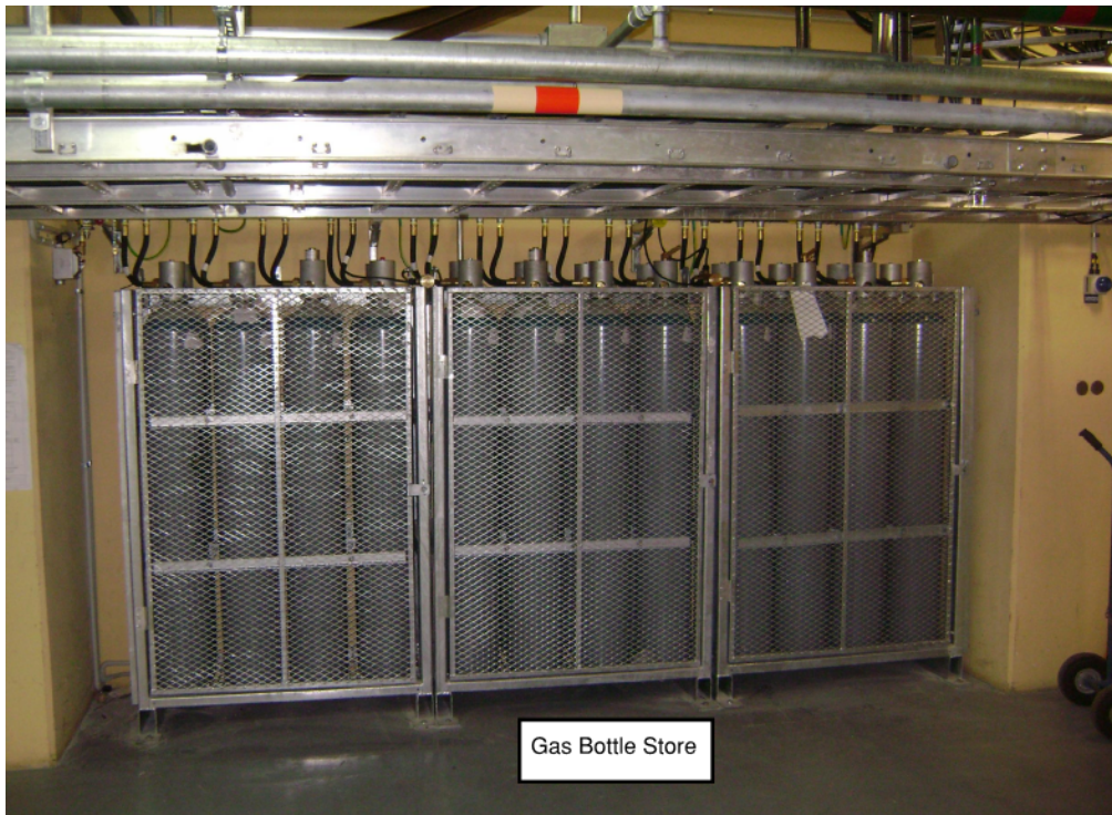
Figure 6 IG-541 Ohau A power station cylinder bank showing cylinder cage modules
